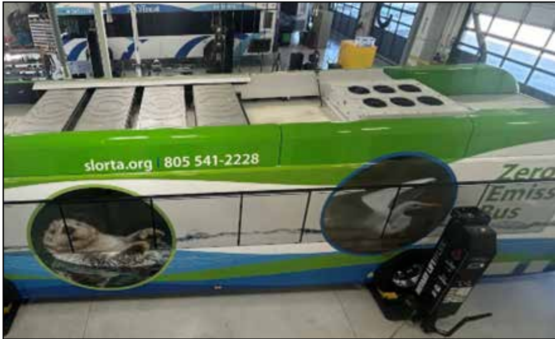
A view of the roof and four battery packs
